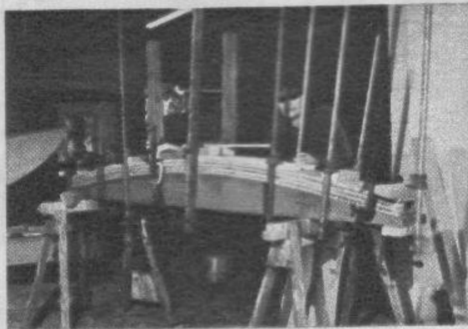
CURVE-CUT two 1x8s, with 2-in. spacer, to make form for laying up front cross beam.
