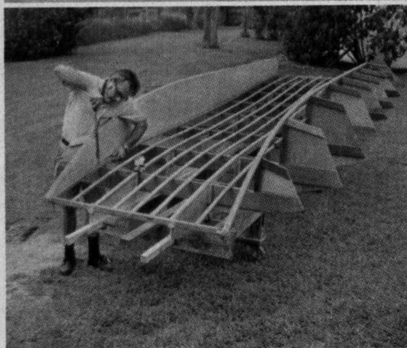
SPONSON inside planking. It's 1/4-in. plywood, glued and nailed to the top batten.
