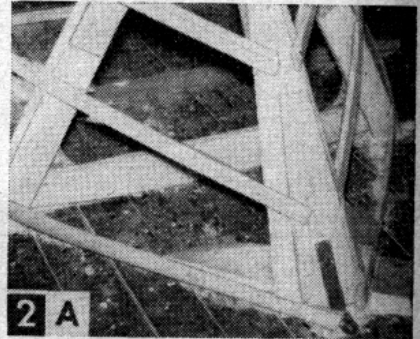
Edges of upper stem are beveled to angle of planking and notched for chine and sheer.
